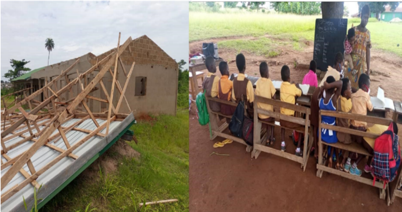
Collapsed roofing, as a result students are studying under trees
