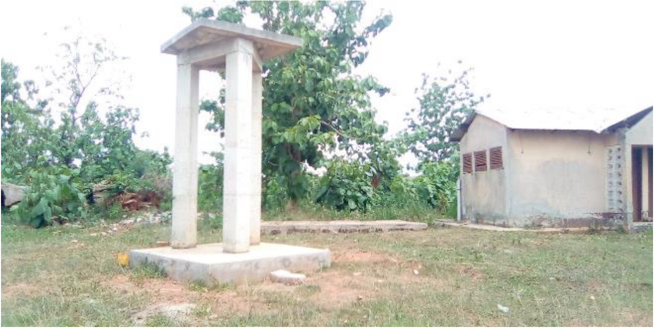
Poly Tank stand for water supply to the toilet facility
